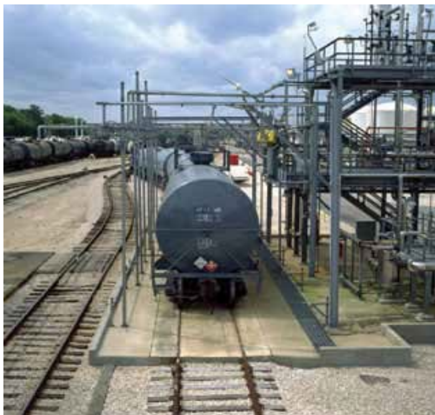
Figure 6.13 EO Unloading Facilities
