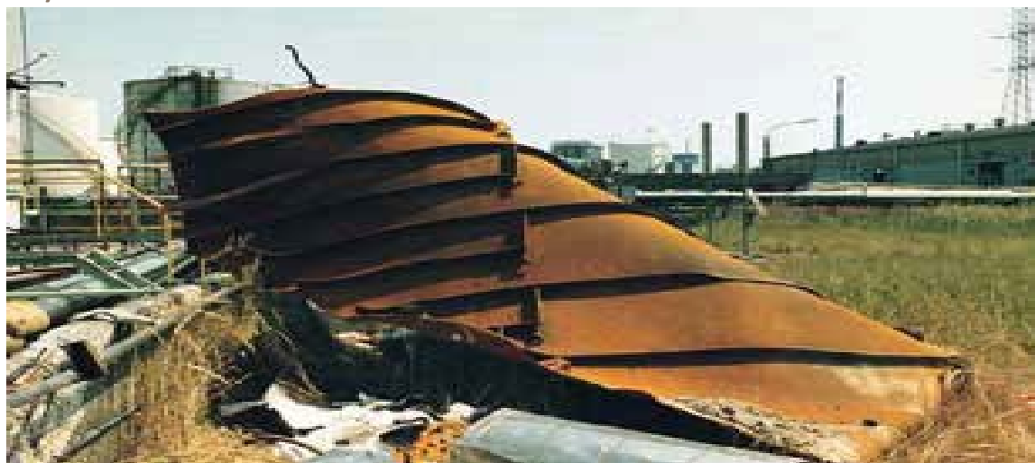
Figure 5.15 Piece of Ethylene Oxide Distillation Column Wall Turned Inside Out by Explosion Hazards of Ethylene Oxide
