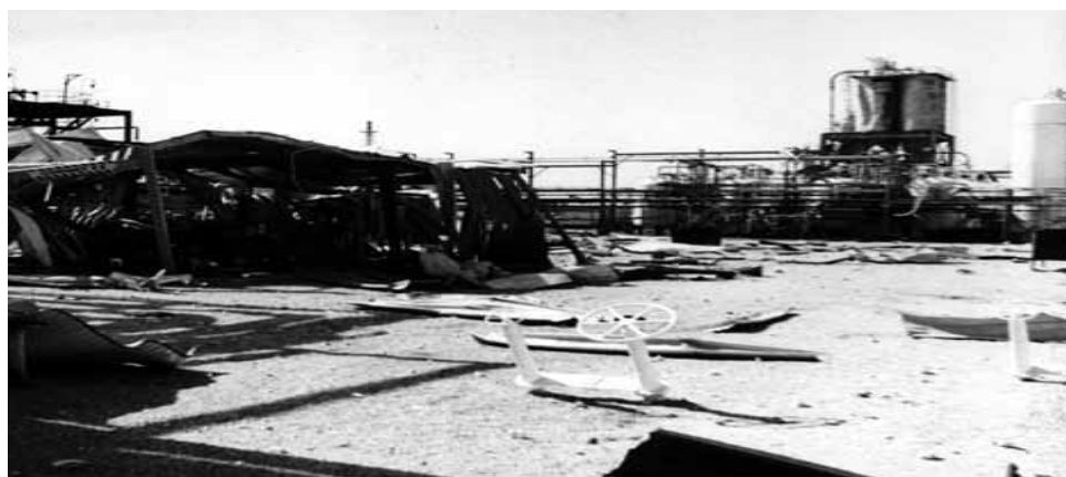
Figure 5.20 Resulting Damage to the Plant
