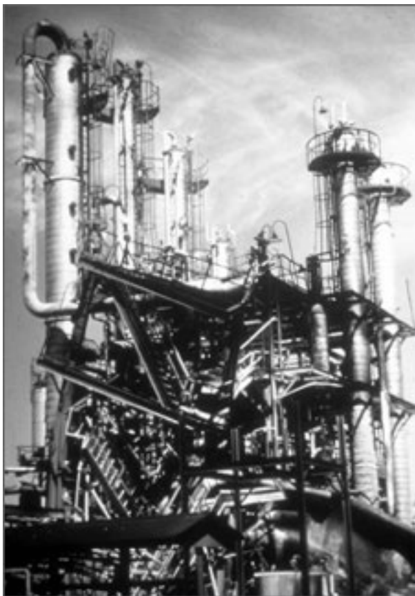
Figure 5.4 EO Tank Blown Into Process Structure 400 Feet Away
