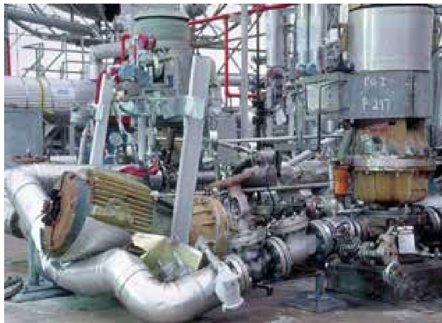
Figure 5.11 Motor Landed on Operating Ethylene Oxide Pump Discharge Line
