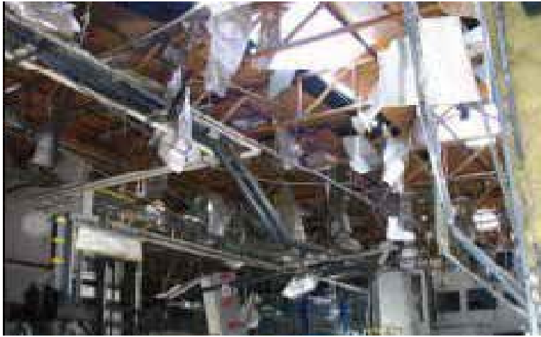
Figure 5.26 Sterilization Chamber Damage
